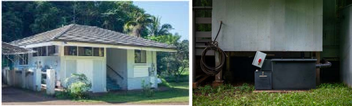
FIGURE 2.2: Site 1 household with 1 bedroom with 2 occupants (left) and mata installed to receive kitchen and toilet blackwater (right).
