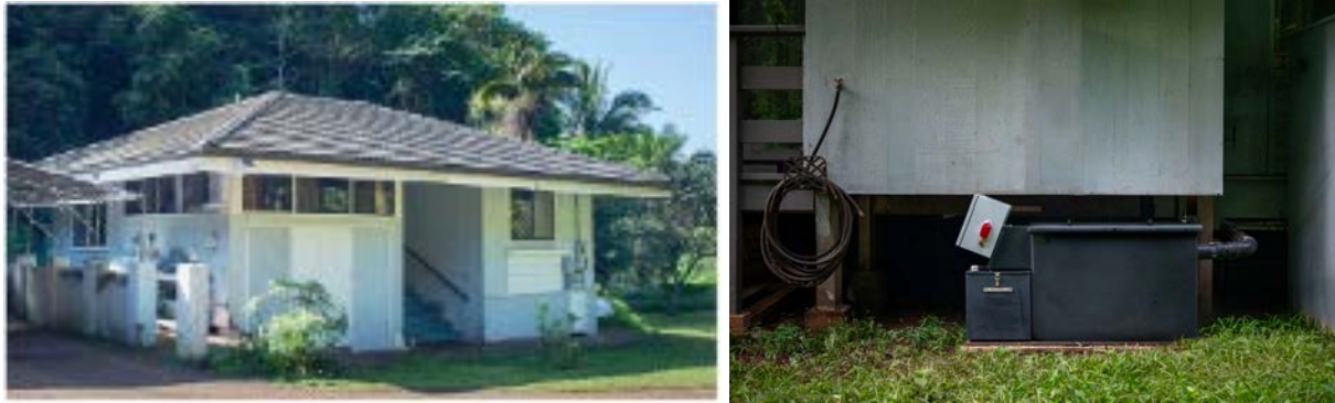
FIGURE 2.2: Site 1 household with 1 bedroom with 2 occupants (left) and mata installed to receive kitchen and toilet blackwater (right).
