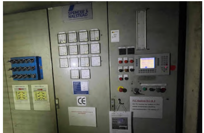
Shot Blasting System (1995) Spencer & Halstead 12 Wheel Monorail
