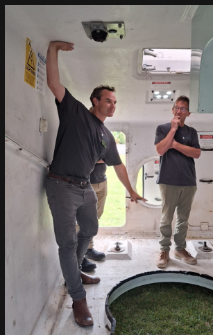
The Armatec Environmental team inspect the inside of the narcelle. They later shared their design insights with participants.
