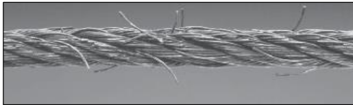
Cable with Corrosion
