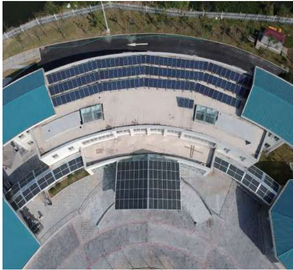
► 54.5KW PV Station in Nantong, China
