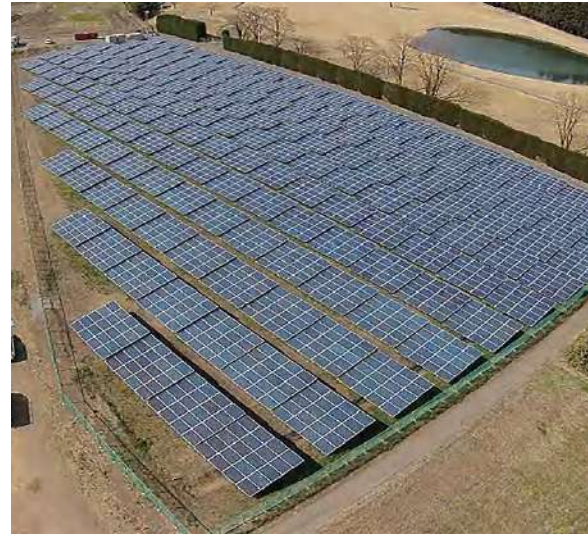
► 875KW PV Station in Takasaki, Japan
