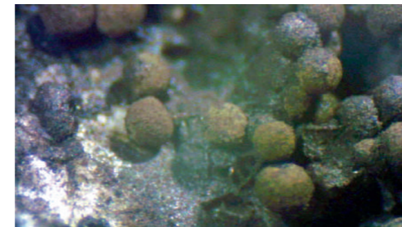
The development of black mould, regarded by hygiene experts as highly concerning, marked the beginning of the end of the trial.
