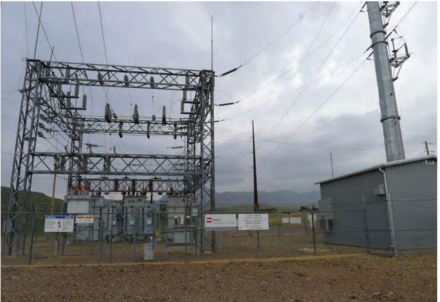
Figure 5: Shafter Mine and Processing Substation.
