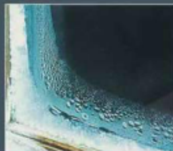
Window condensation can fuel mold growth
