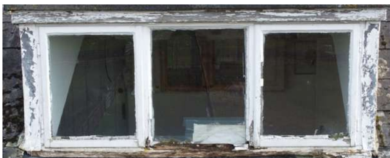
Rotten windows in the main house
