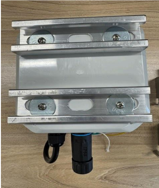
Relay Box secured to aluminum channel with 10-32 bolts & 3/16" washers
