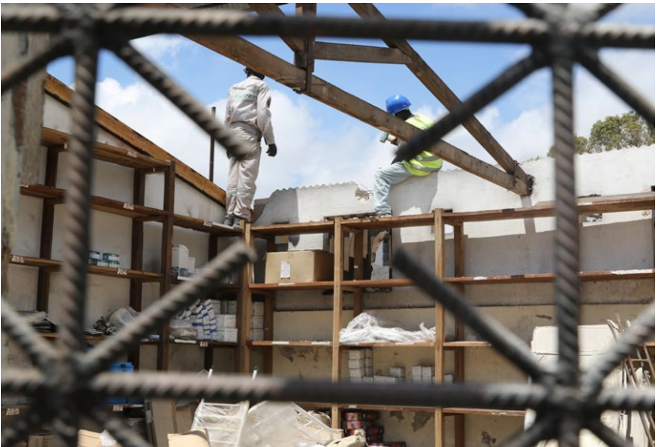
Cabo Delgado Province. The ICRC helps with the repair of the roof of a health centre. The roof was destroyed when Cyclone Kenneth struck in April 2019, Mozambique. Image: Nxedlana, Khatija/International Committee of the Red Cross
