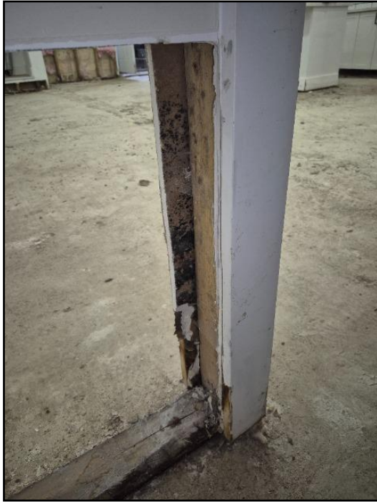
Drywall/insulation/vapour barrier cut back...
