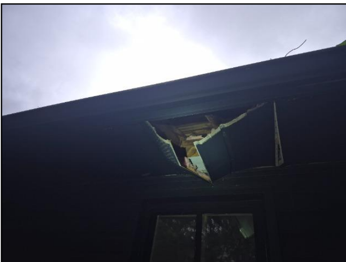
Loose or missing pieces
