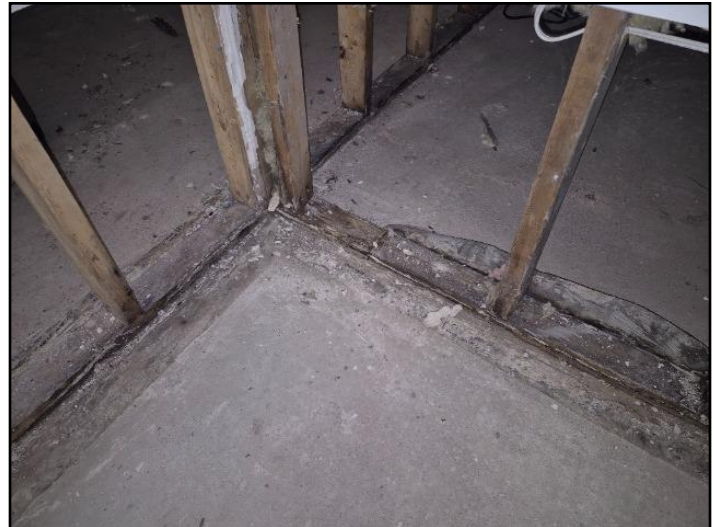
Drywall/insulation/vapour barrier cut back...
