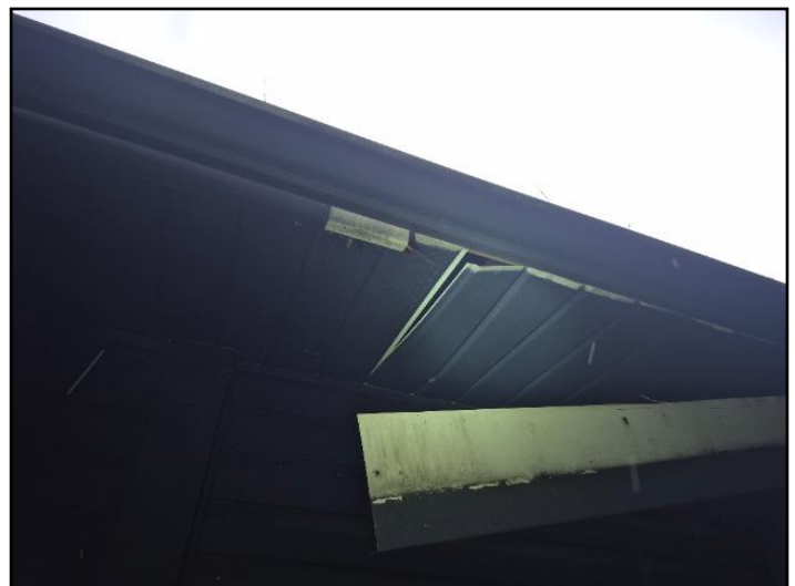
Loose or missing pieces
