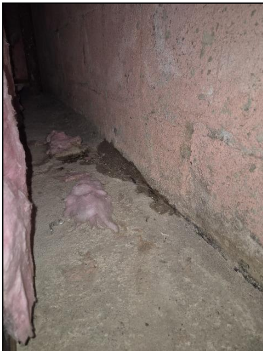
Drywall/insulation/vapour barrier cut back...
