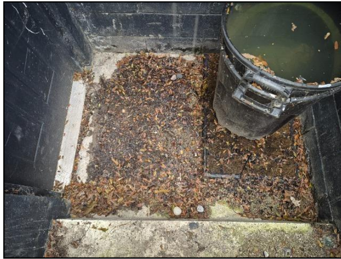
Drains missing, clogged or undersized
