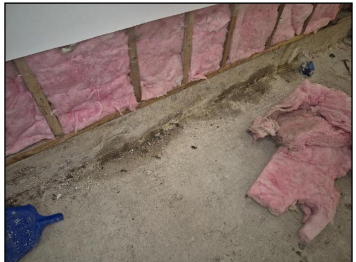
Drywall/insulation/vapour barrier cut back...
