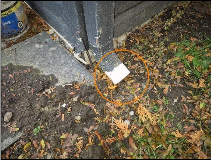
Discharge too close to building
