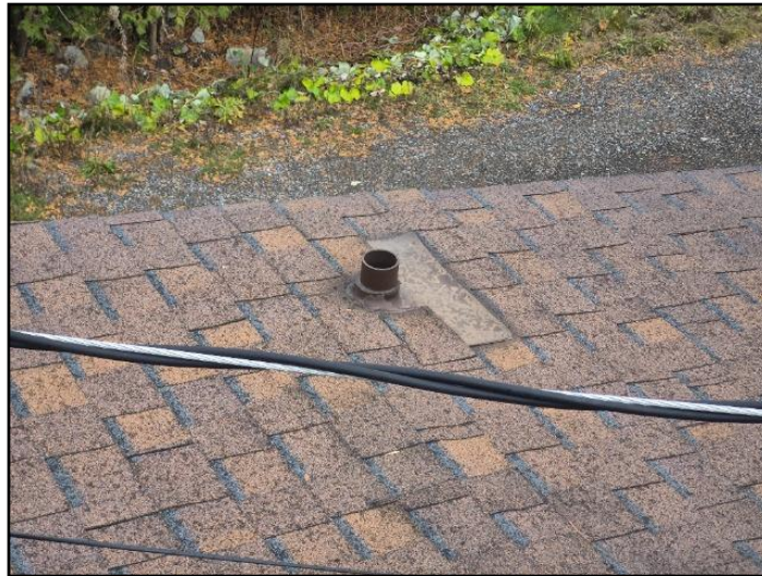
Vent termination problems
