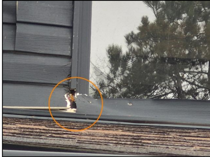
Damage, loose, open seams, patched
