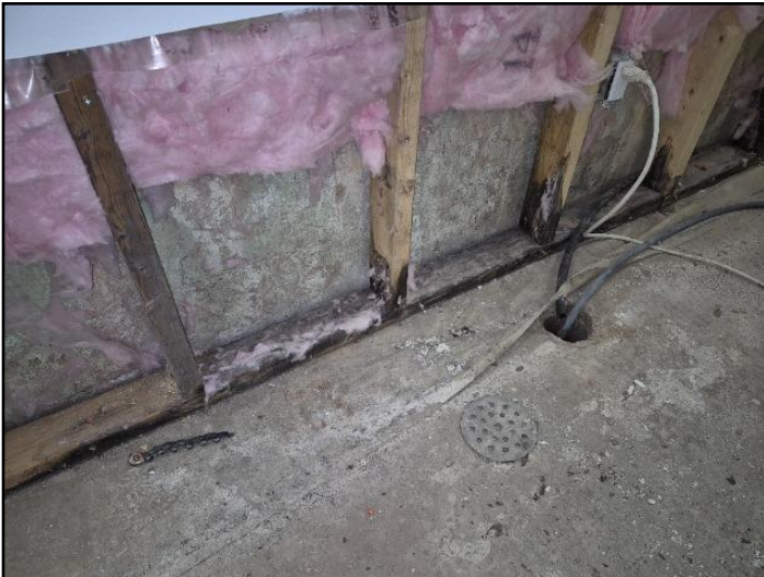
Drywall/insulation/vapour barrier cut back...
