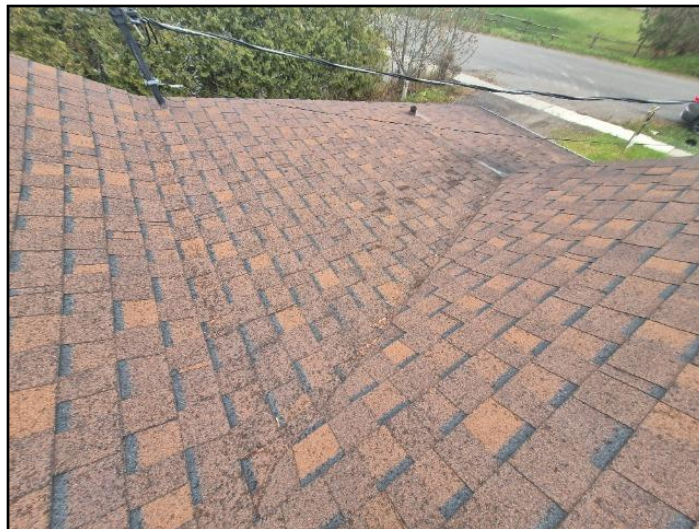
Slope too low
