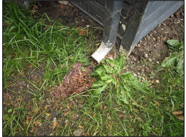
Discharge too close to building
