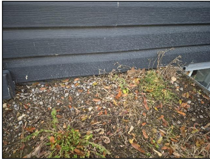
Too close to grade
