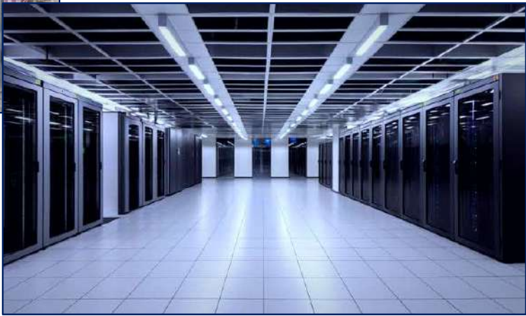
Inside a modern AI Datacenter
