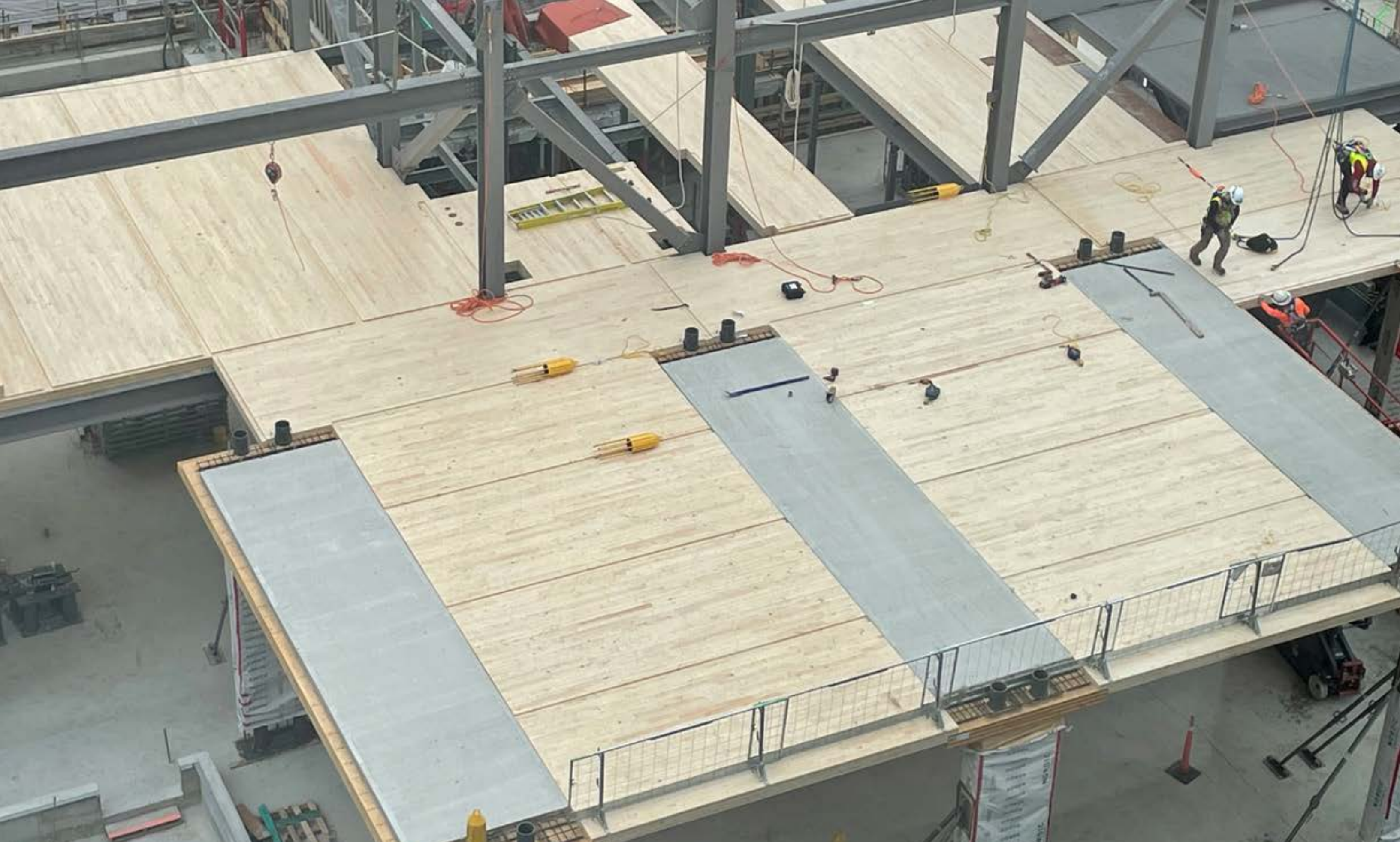
AERIAL VIEW OF THE GLULAM COLUMNS, CLT SLAB BANDS, CLT INFILL PANELS AND STEEL CORE
