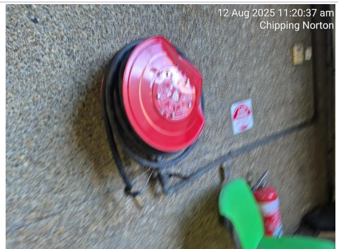
Fire safety equipment
