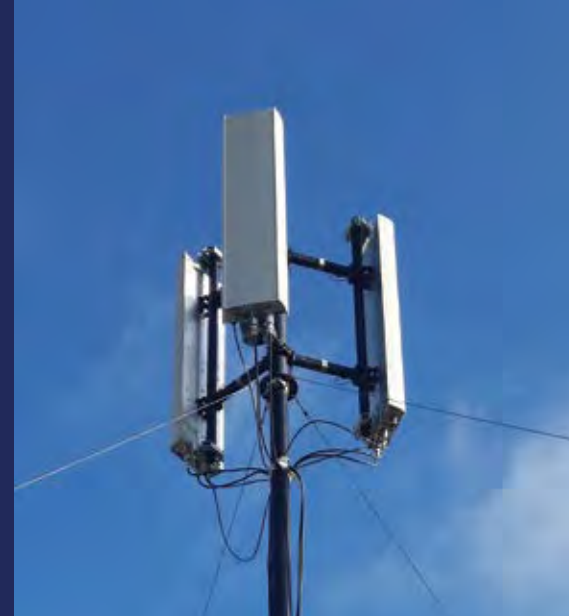
Sector Antenna Array for LTE Base Station System
