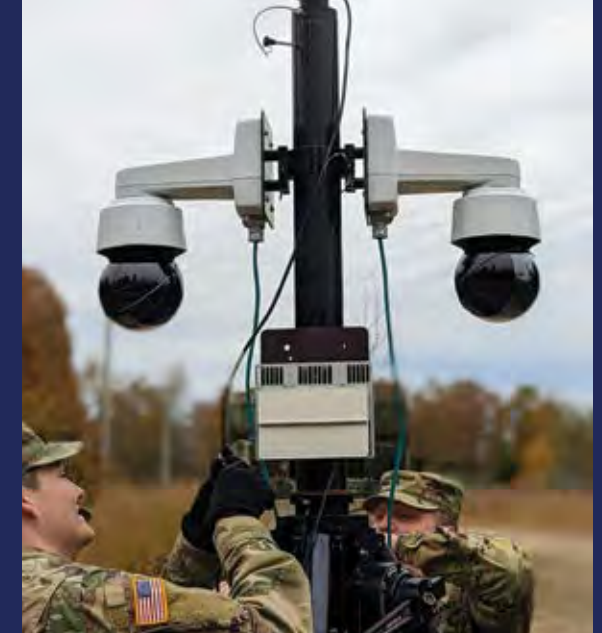
PM / TS Security Surveillance System
