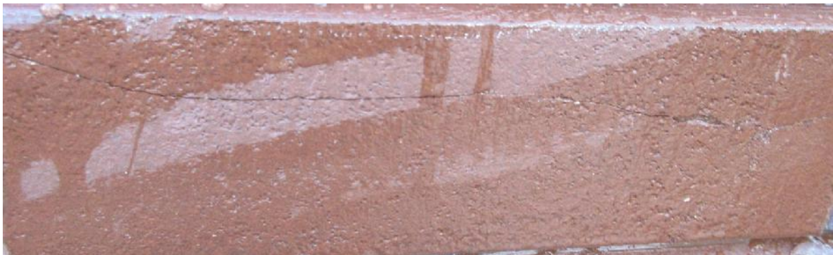
6 Nm HARD BODY IMPACT - CRACK IN BRICK WITHOUT MORTAR
