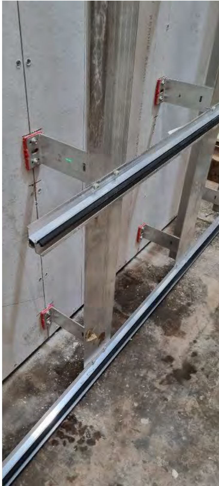
Plate 3 - Application of TI Generic Horizontal Starter Rails for the Bottom Row of Ceramic Panels
