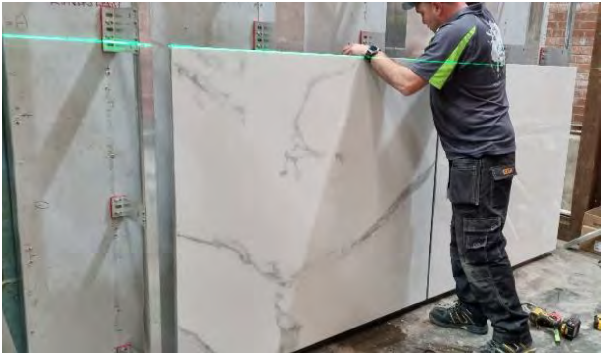
Plate 4 - Installation of the Bottom Row of Ceramic Panels on the Rail System
