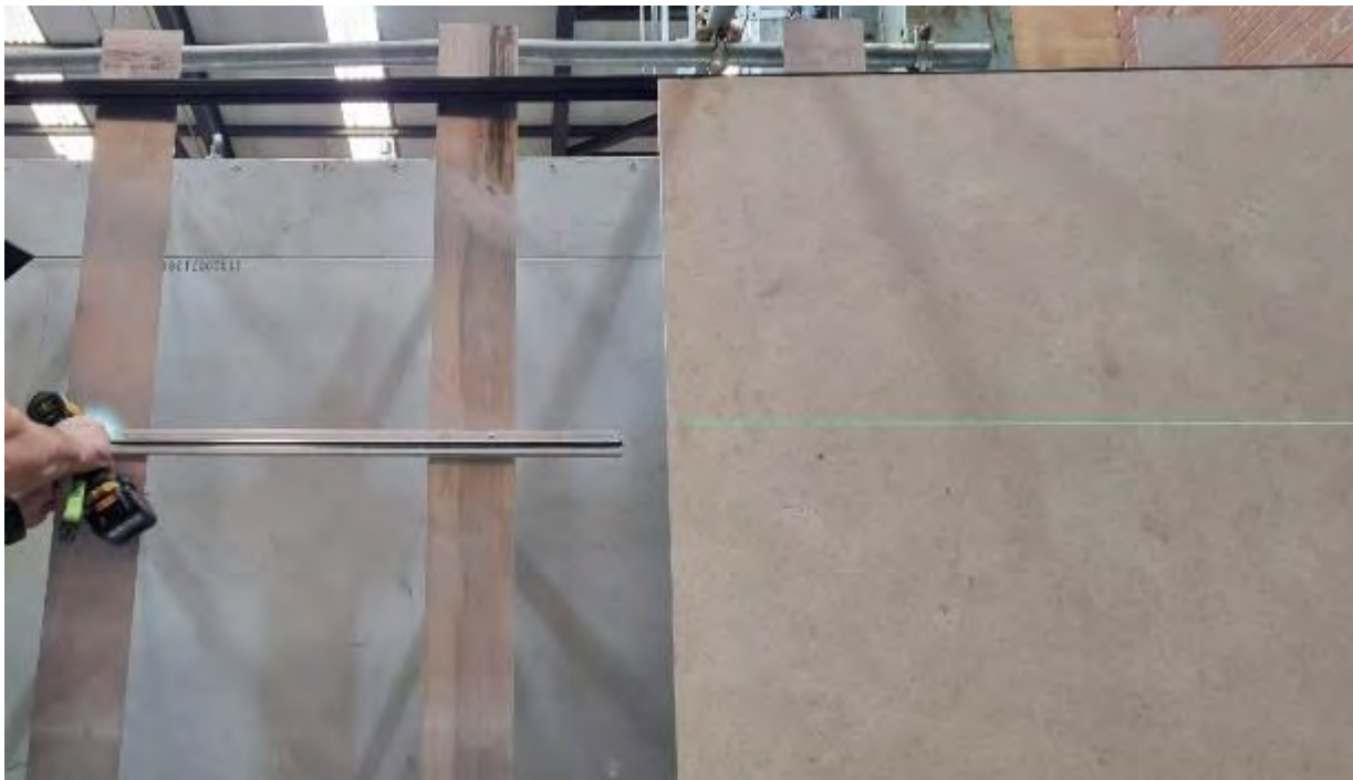
Plate 5 - Installation of the Top Row of Ceramic and Stone Panels on the Rail System
