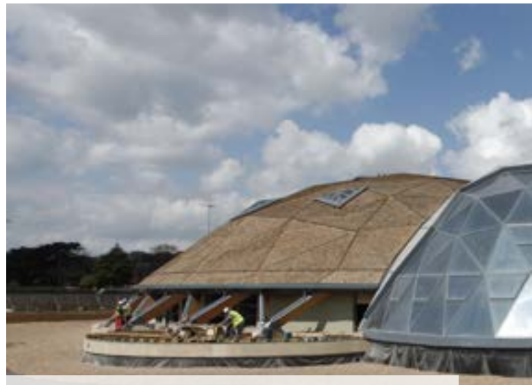
Sport and recreation centre – United Kingdom RENOLIT ALKORPLAN Solar profiles as basis for mounting cedar shingles and aluminium panels.
