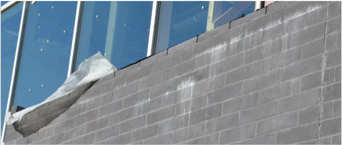
Top of wall protection partially removed by roof contractor prior to permanent coping installation - note efflorescence formation
