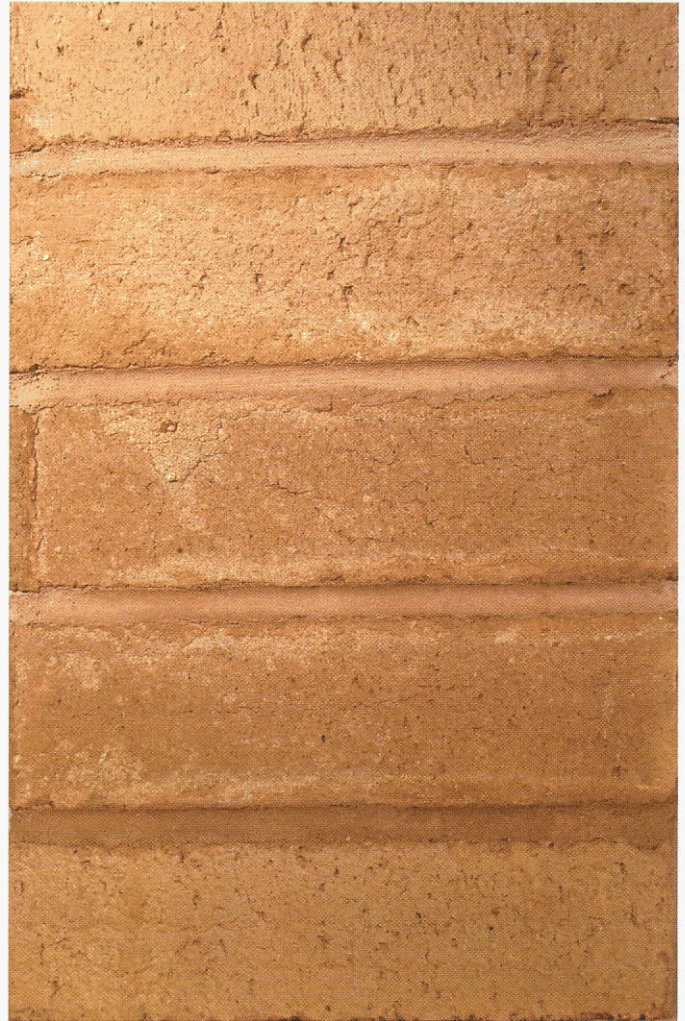
Fig. 3. In this example, a masonry prism was constructed using one batch of mortar. The top mortar joint was tooled immediately after placement of the unit. Remaining mortar joints were tooled at progressively greater time intervals and thus stiffer consistency. The relationship between mortar consistency when tooled and mortar color is quite apparent.
