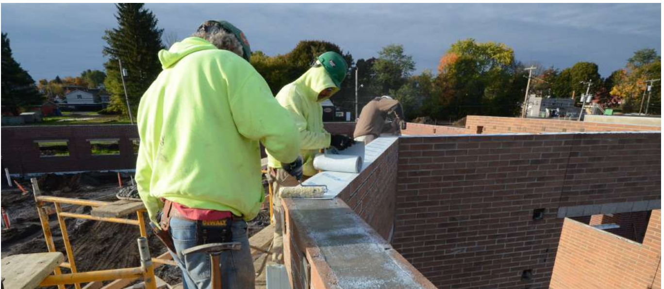
Adhering a water resistive membrane to the top of the wall – this can be left in place when the roof is installed
