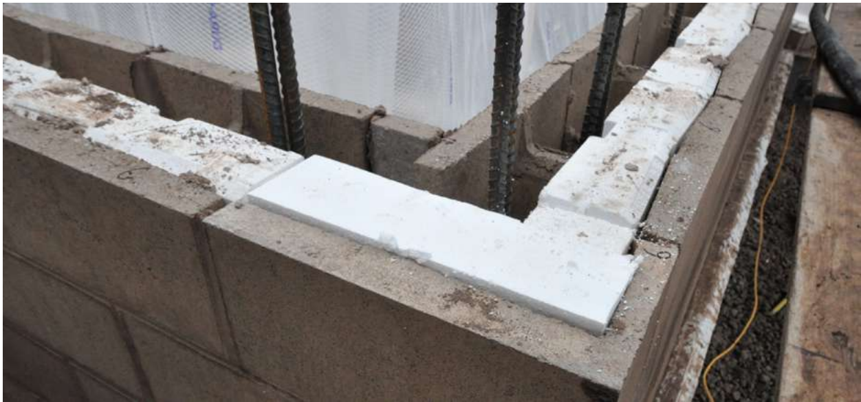
Corner Detail with L-Shaped Fitting Cut from 8x8x16 Jamb Unit with EPS Insulation Cut to Fit
