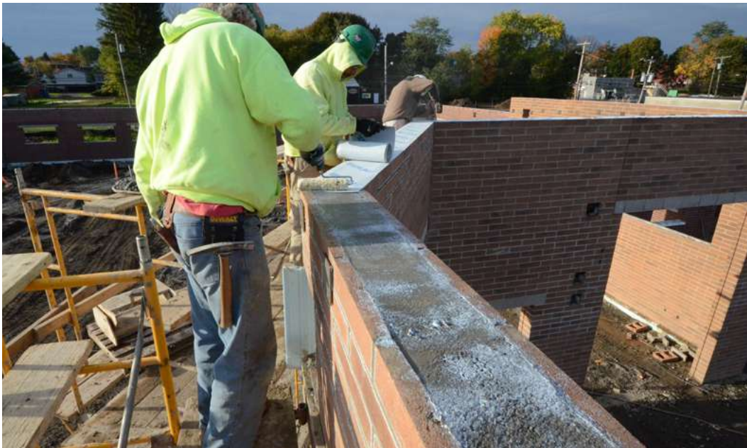
Protective covering prior to permanent capping of the wall This is also done by securely tarping the wall top
