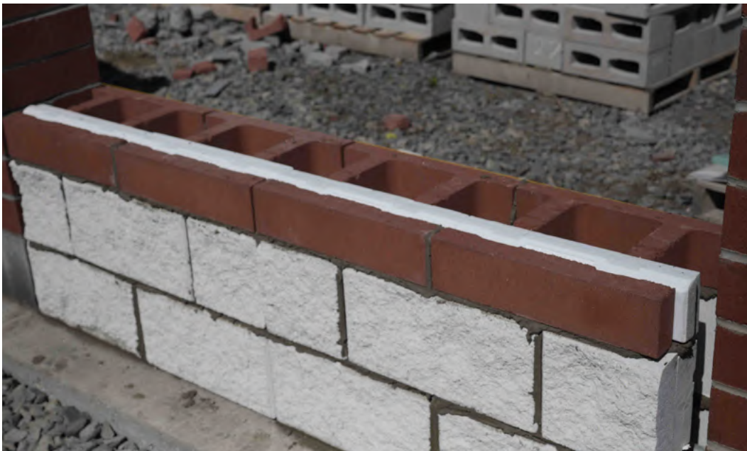
HI-R and HI-R-Half High wall under construction (shown prior to tooling joints)
