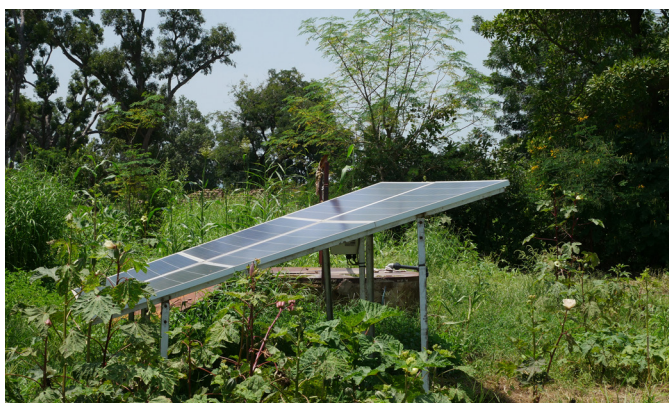
Solar water pumping system Photo: DEM
