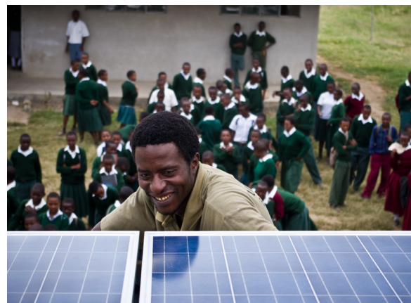
Solar photovoltaic installation at a school Photo: DEM
