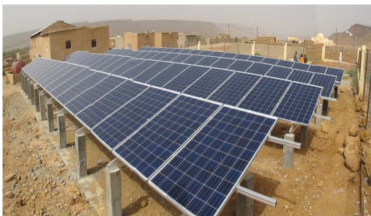
Solar Photovoltaics Photo: Danish Energy Management (DEM)
