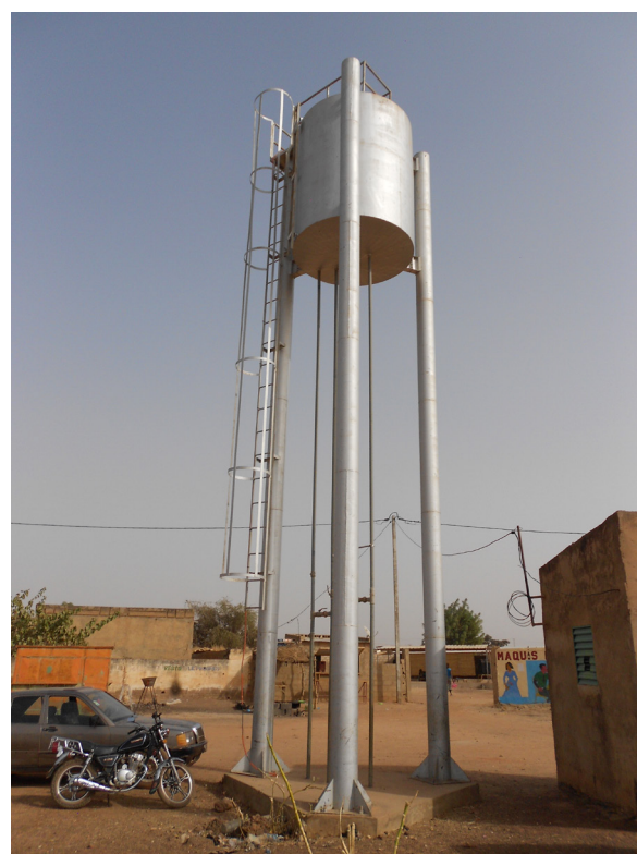
Solar photovoltaic water pump Photo: DEM
