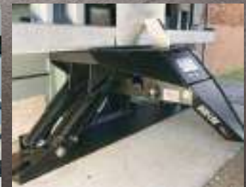
Stabilizing Trailer Restraint with cover plate obstruction
