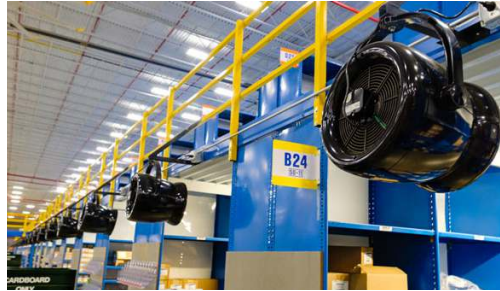
Spot Cooling Application
