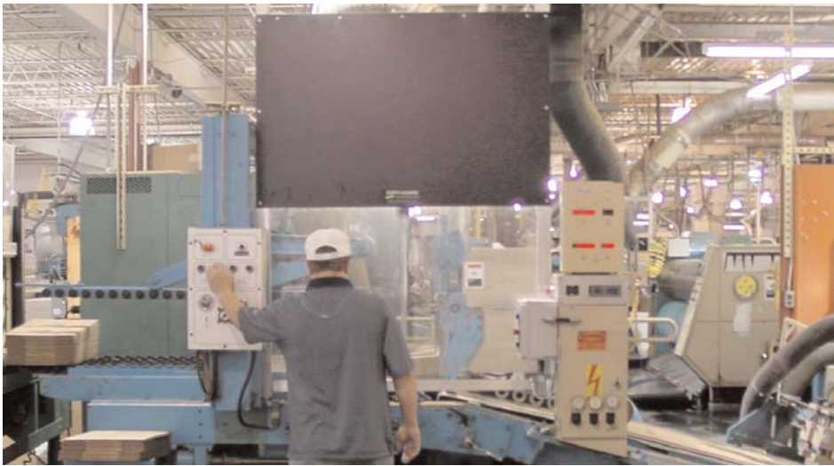
The automated Verti-Guard barrier from Frommelt Safety Products protects employees from the hazards of the flexo-folder-gluer machine, yet allows full visibility of production process.
