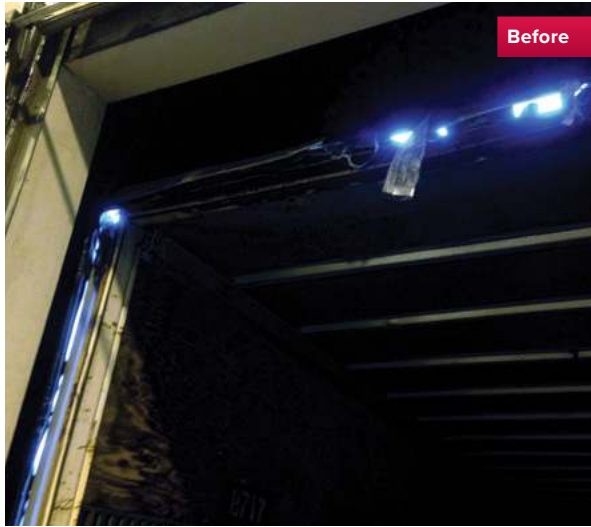
Gaps at top and corners of head curtain
