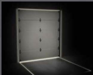
Leveler and door gaps
