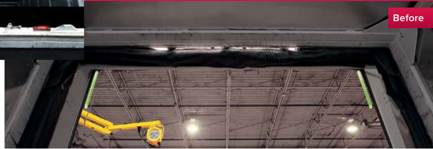
Gaps from trailer protrusions in dock seal header
