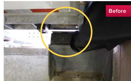
Gaps at raised bumpers
