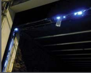
Top and corner gaps
