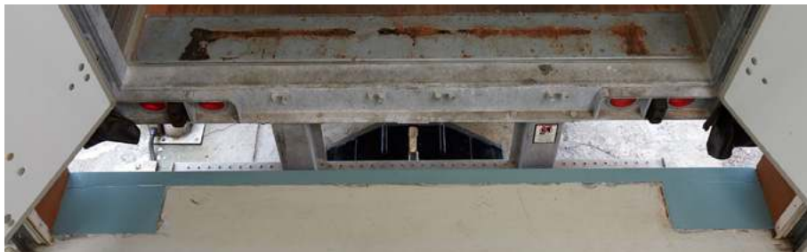
Open gaps between the dock face and trailer allow contamination, infiltration, and increased energy costs
