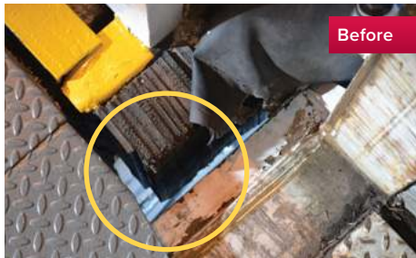
Gaps around bumpers
