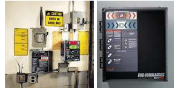
Multiple controls at each dock position can be complicated and potentially dangerous.
