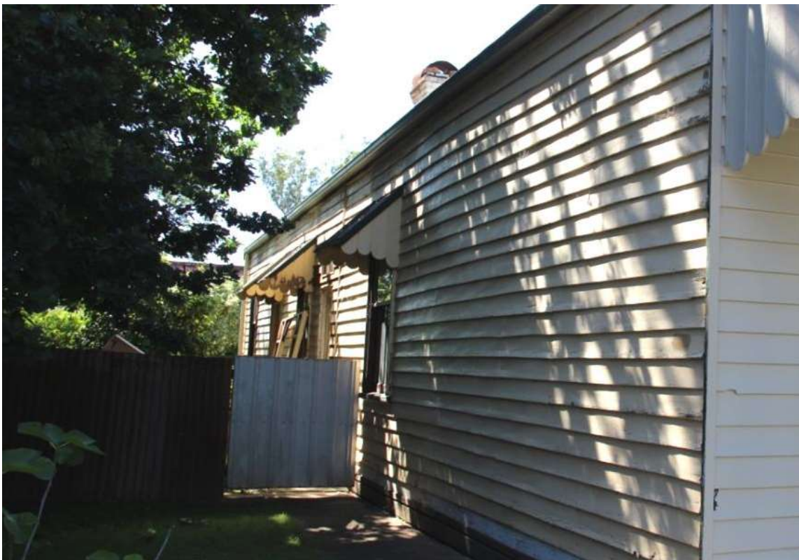
Figure D2. The north elevation has openings to the rear of the building, including three with skillion-roof hoods and round-edged cladding to the sides, like the verandah. One has since been rectified by owner, due to severe rot (Feedback from owner 9 May 2016).
