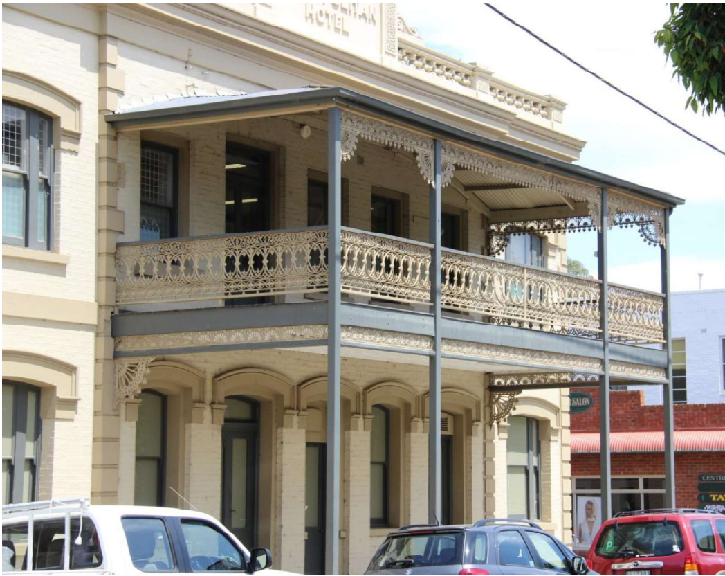
Figure D5. The many openings to the facade (except those under the verandah on the first floor) have bold segmental-arched mouldings to the top and are recessed within rendered surrounds. All windows have timber-framed one-over-one sash windows. The verandah posts are not original.
