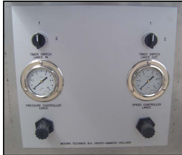
Pressure, Speed Controls and Switches (Outside Panel of Cabinet)
