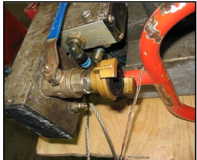
2TLE – Air Hose Connection
