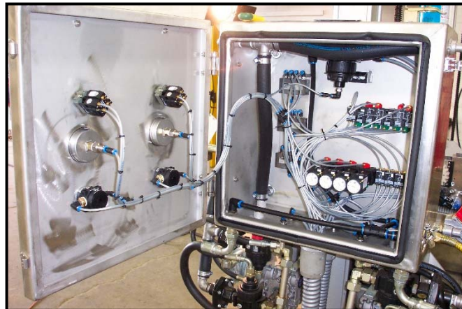
Cabinet Control Switches (Inside Cabinet)
