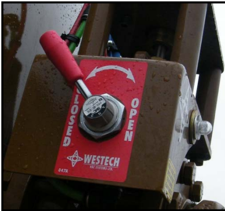
Valve in “Closed” position
