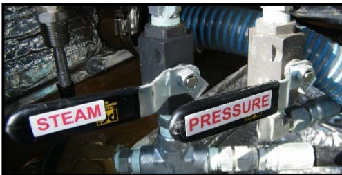
Steam/ Pressure Gauge
