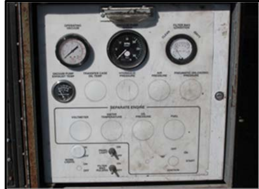
Hydraulic System Control Gauge Panel
