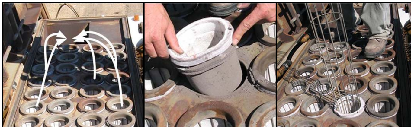
A View from top of unit with bag house door open
