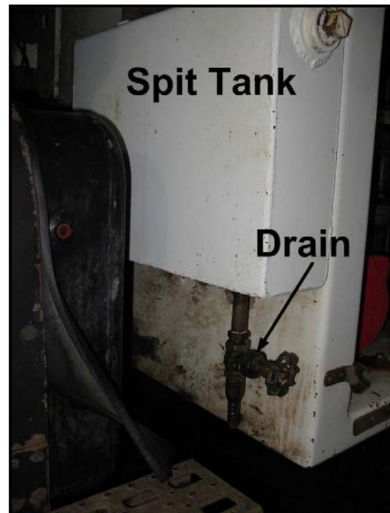
Spit Tank and Drain
