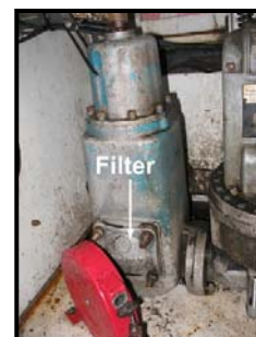
Strainer Filter Location
