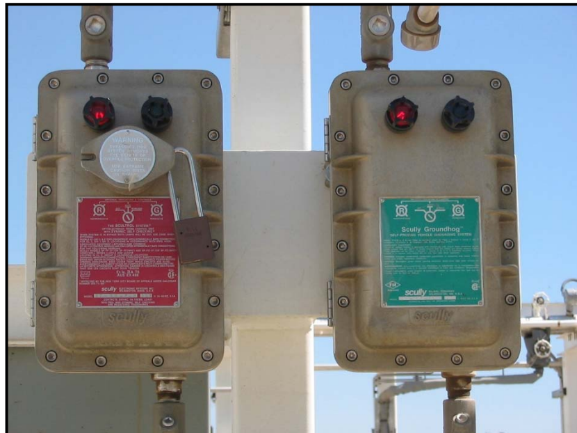
Ground Indicator and Scully Indicator – Both indicators are red
