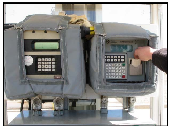
Operator Activating Control Panel
