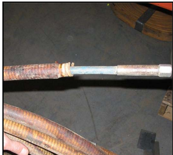
High Pressure Water Line that has been removed from service
