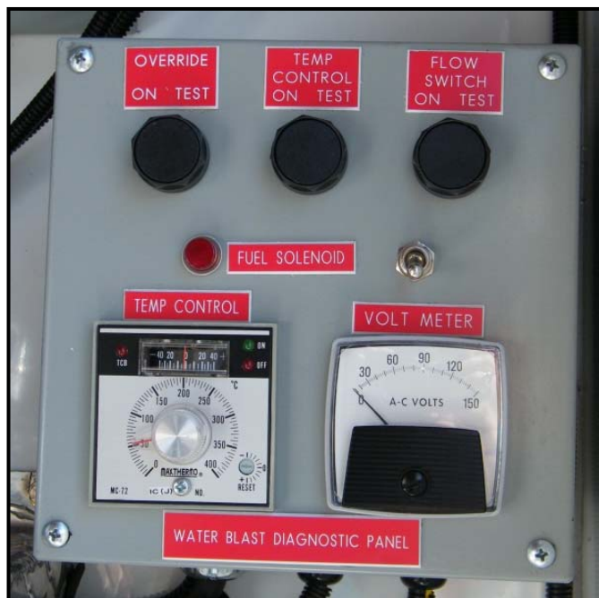
Boiler Control Panel
