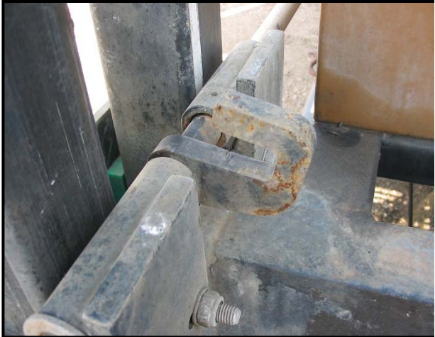
Locking Bracket Used to Secure Cabin Frame in Raised Position
