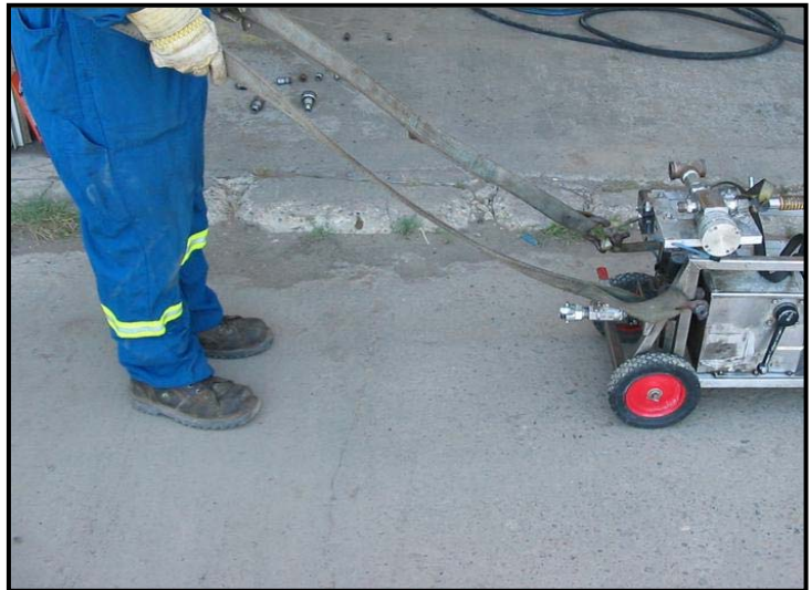
Technician Reversing Roto Fan Twister
