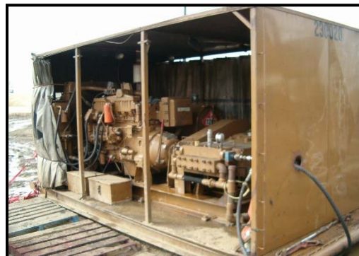
One Pump in a dual pump system
