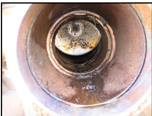
Air Actuated Valve Partially Open
