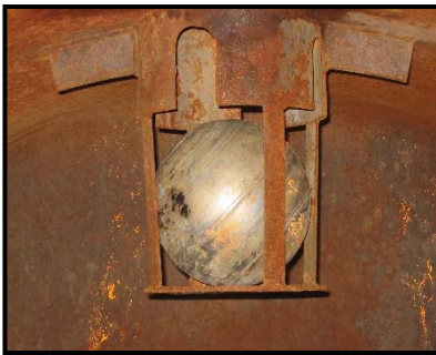
Overflow Shut-Off Ball and Basket
