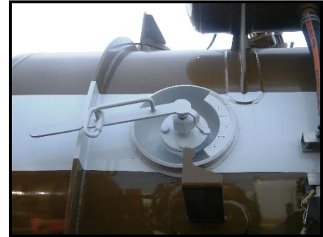
Exterior Tank Level Indicator
