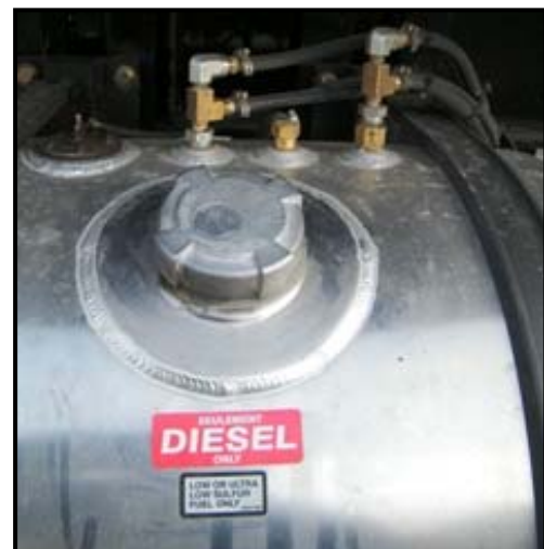
Auxiliary Diesel Tank
