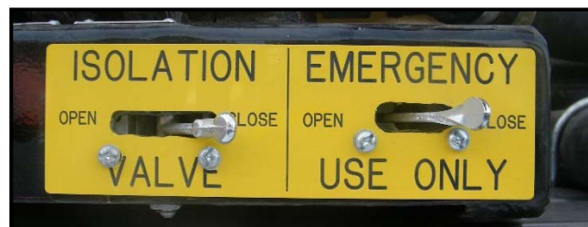
Isolation Valve and Emergency Use Only Switches
