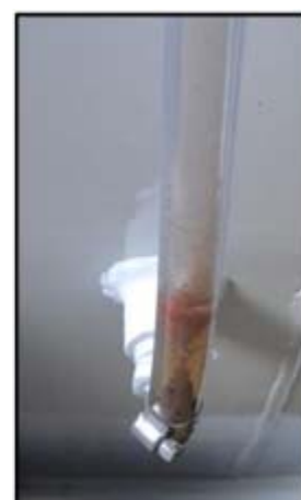
Sight Gauge Close Up
