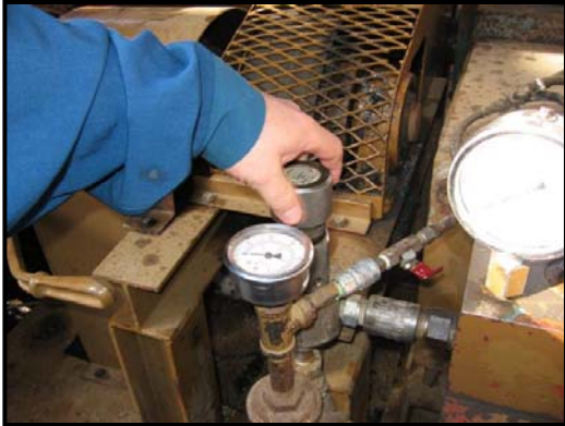
Valve, Needle Valve, and High Pressure Gauges
