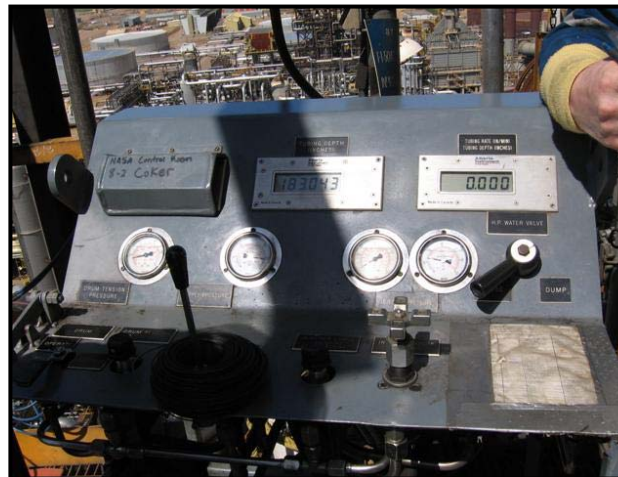
Operator Panel (with controls, digital pressure and distance displays)
