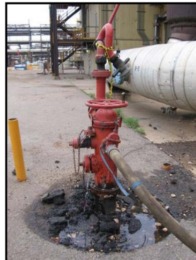
Fire Hydrant (with attached water (fire) hose)
