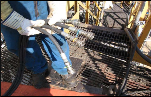
Hydraulic Hoses before connection to Control Panel
