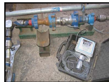
"T" Valve with Flow Meter connected
