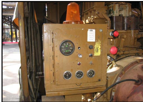
Pump Control Panel
