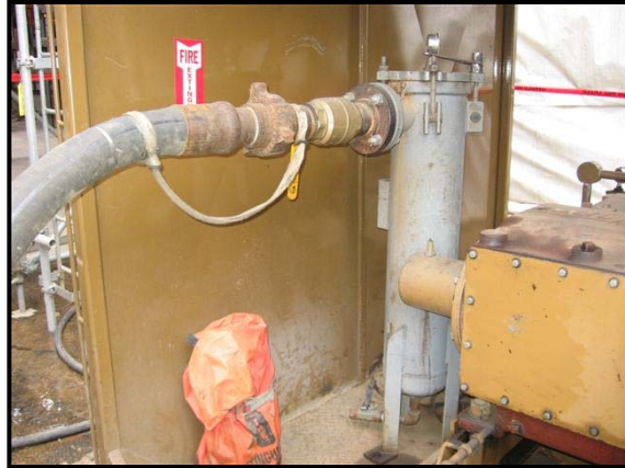
High pressure water line (with whip check exiting pump on left)
