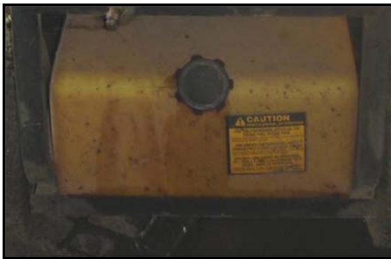
Fuel Oil Tank
