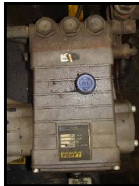
Water Pressure Pump
