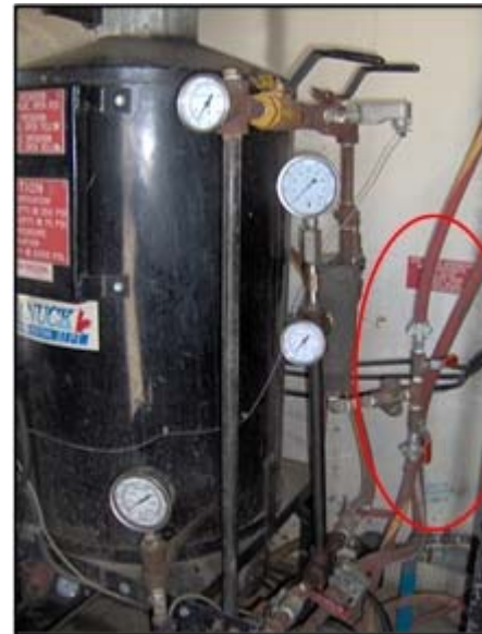
Dry Steam Operation Panel - Hot Condensate
