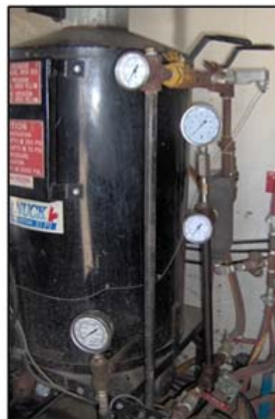
Pressure & Temperature Gauges
