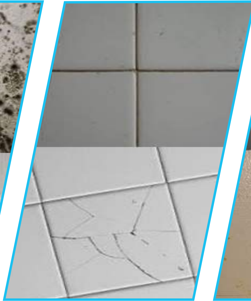
Tiles – Grout Lines & Breakage
