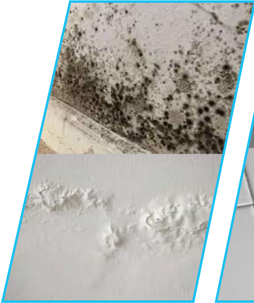
Painted Walls - Mould & Flaking
