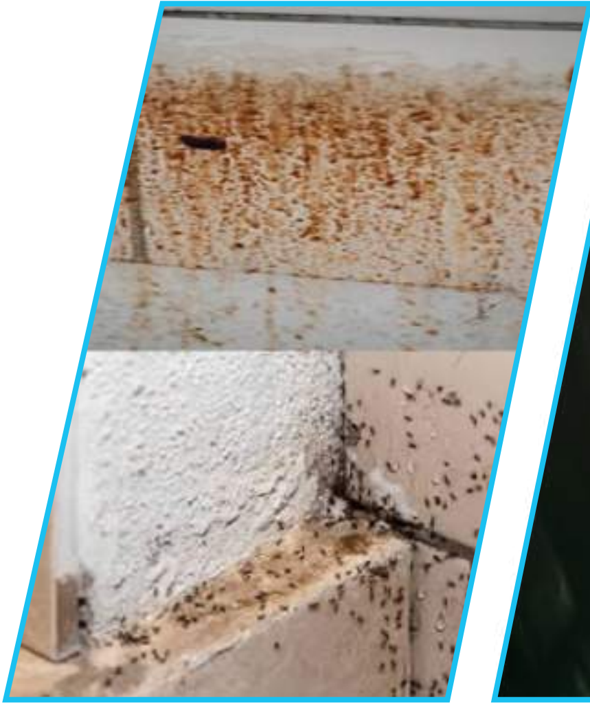
Oil Stains & Infestation
