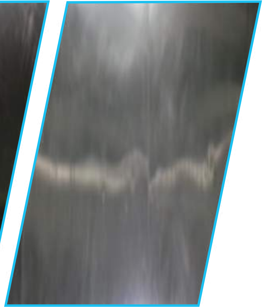
Metal Cladding – Cleaning Issues
