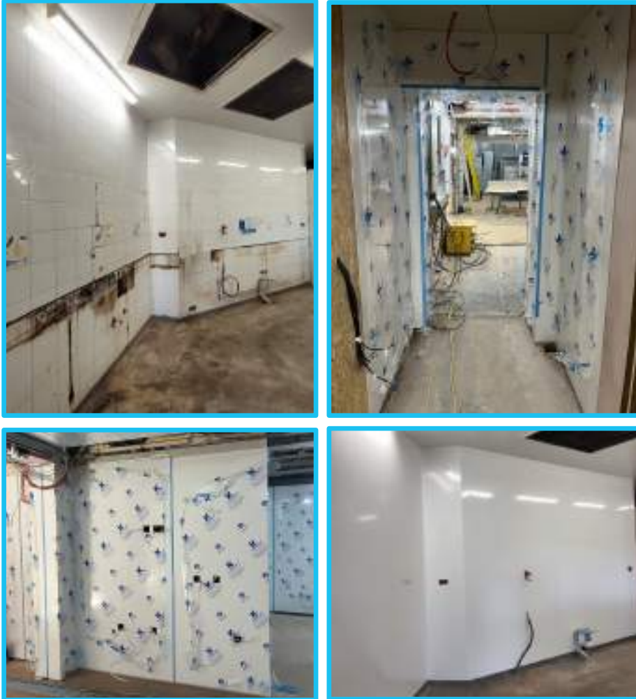
Commercial Kitchen Project : Stoke, U.K.
