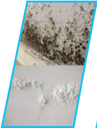
Painted Walls - Mould & Flaking
