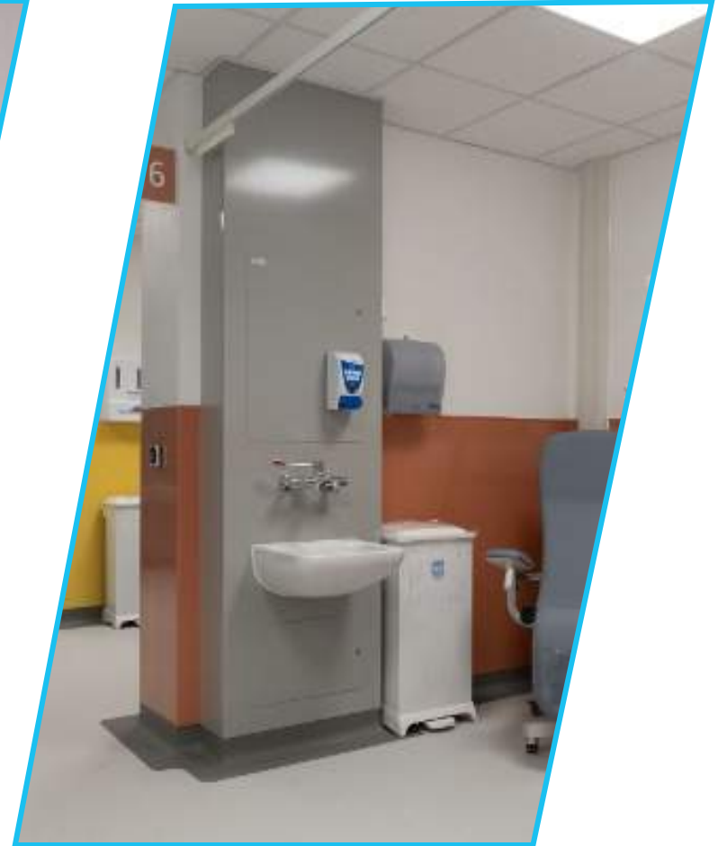
Integrated Plumbing Systems (IPS)
