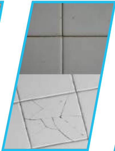
Tiles – Grout Lines & Breakage
