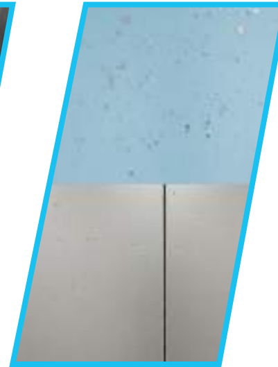
Metal Modular – Paint Peel Off & Denting
