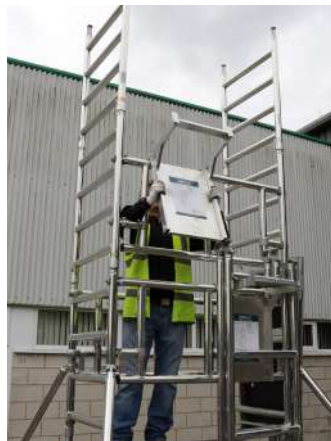
24. Relocate the side “empty” assembly bracket on the front of the tower (top rung of the tallest guardrail frame as shown).
