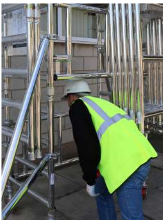
20. Access the platform by passing under the side frame and via the trapdoor platform.
