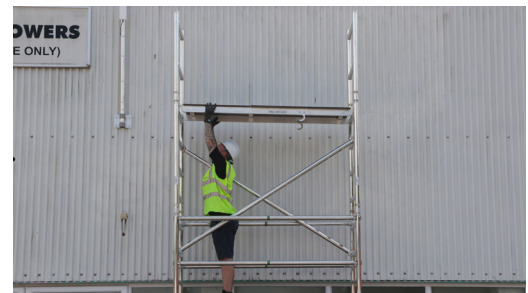
10. Fit your next trapdoor platform to the 3rd rung down from the top. This will be the top rung of your TT4F.
