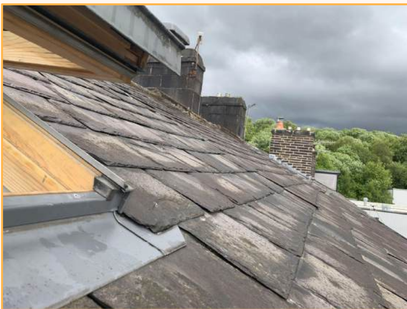
Roofs on back to back homes are shared with neighbours on either side and also to the rear. This can add complexity to retrofit projects - especially where roofs feature dormers and rooflights.
