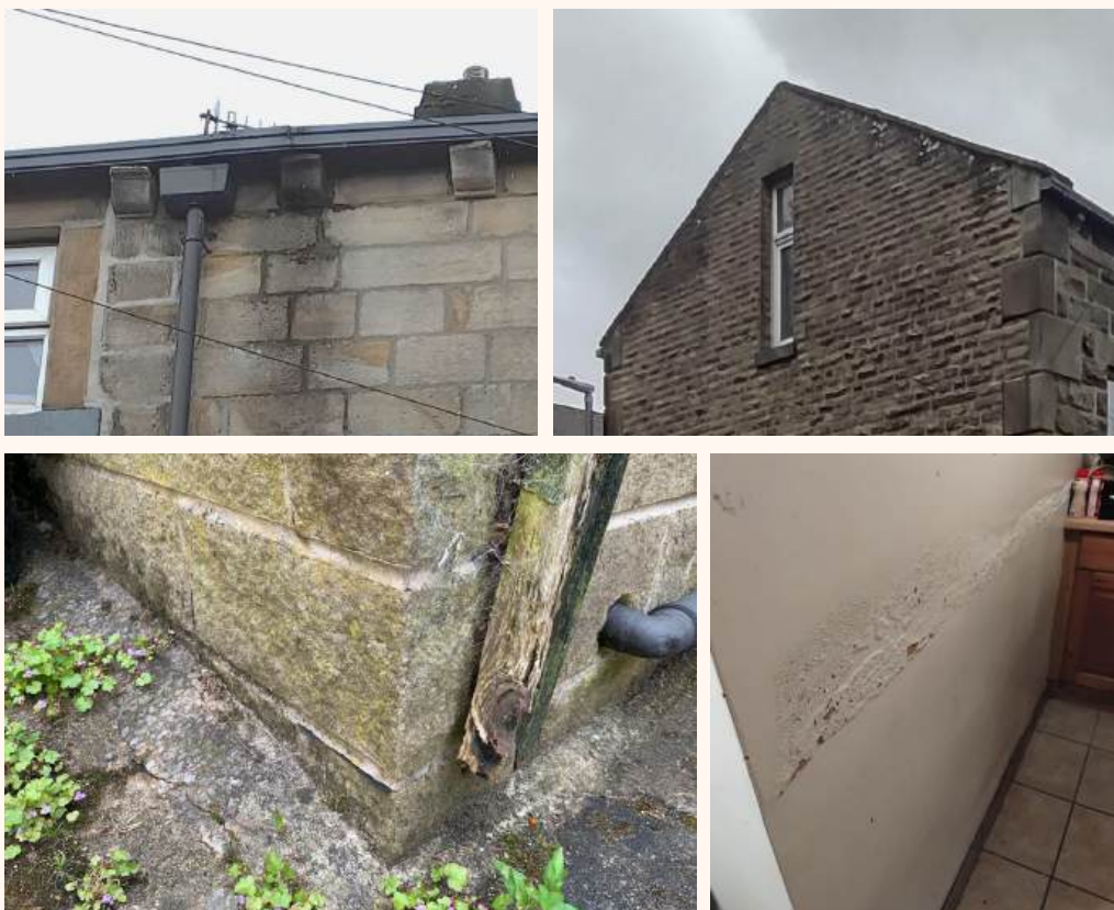
Images clockwise from top left: 1. A gutter joint with a leak where a new and old gutter meet, causing dampness in the stone wall. 2. A clipped verge - the edge of a roof at the gable - showing staining where wind driven rain is making the wall damp. 3. Evidence of high levels of moisture in walls at ground level where rain hits paved areas and bounces up onto walls. 4. Areas of damp on internal walls caused by poor drainage at ground level where walls are partially against the ground.
