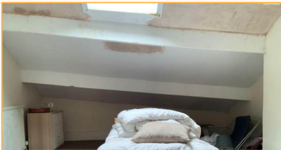
Photo showing the complex roof geometry in the attic of some terraced homes.
