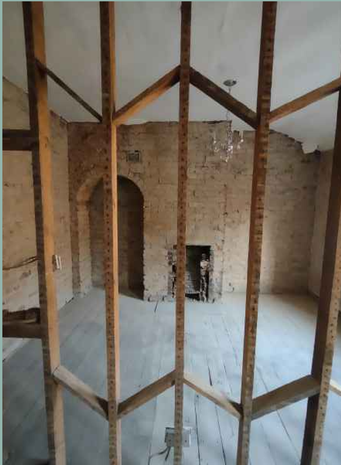
Stripped back Saltaire bedrooms with original partition wall ready for internal insulation.
