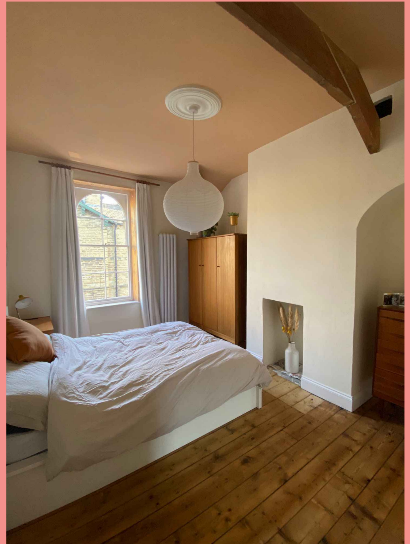
Saltaire room with internal insulation applied to the outside wall and chimney breast.
